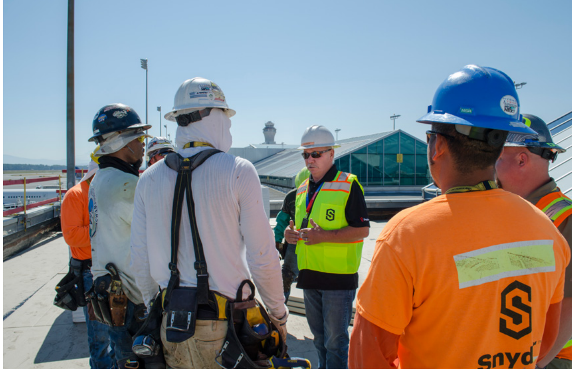
Nicolai talks to the roofing crew about the plan for the day and answers any questions they may have about their responsibilities, or the site they are scheduled to complete.
